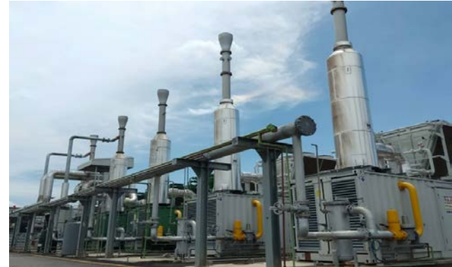
Methane recovery from landfill site for electricity generation by Crane Renewable Energy Co.,Ltd.
