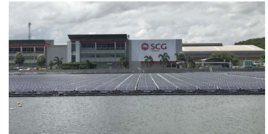
978.75 kWp floating solar farm project on pond of SCG chemicals, Maptaphut Sub- district, Mueang Rayong District, Rayong,
