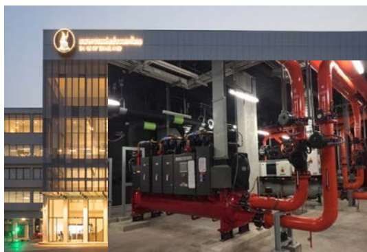
Replacement of Existing Chiller with High Efficiency Chiller By Bank of Thailand Learning Center
