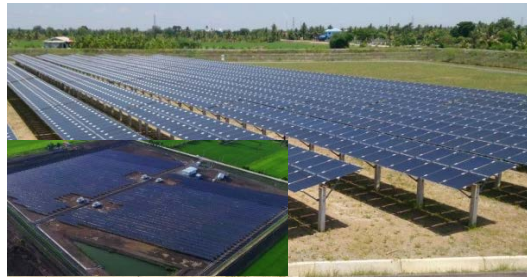
5 MW Blue solar farm 1 power plant
