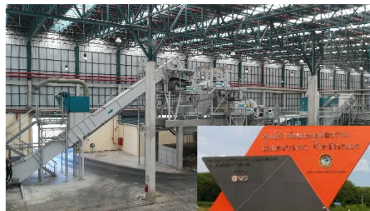
RDF production from municipal waste at Rayong by GPSC
