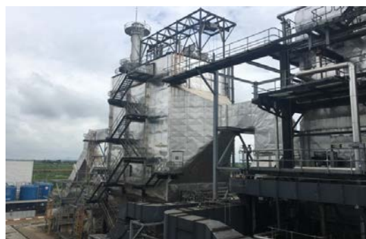
Electricity generation from biomass by Nakornphet Greenergy Ltd.
