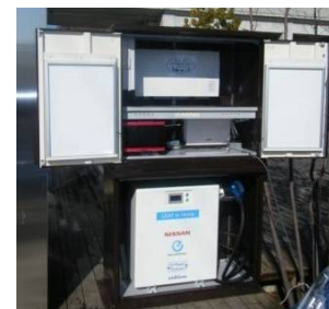
Emergency power BOX
