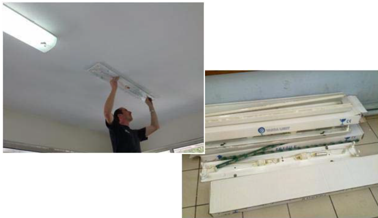
c) Reduction of electricity consumption in municipal lighting
