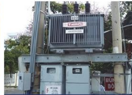
High efficiency transformers in power grids (Viet Nam) 7,972 tCO 2 /y. Start operation 2016-2018
