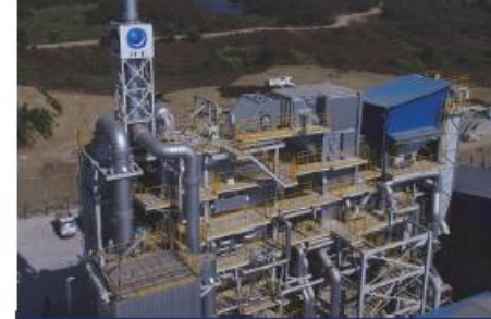
Waste to Energy plant (Myanmar) 4,732 tCO 2 /y. Start operation: Apr. 2017
