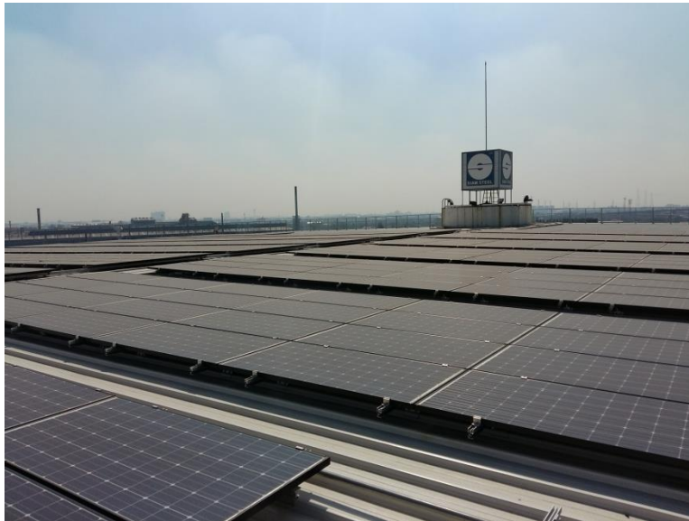
Office building rooftop: 195.84 kW
