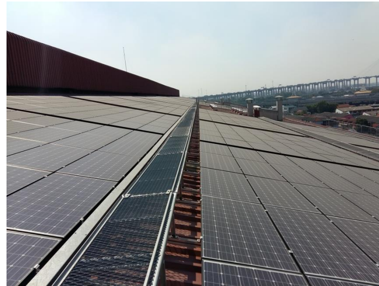
Factory rooftop: 798.72 kW
