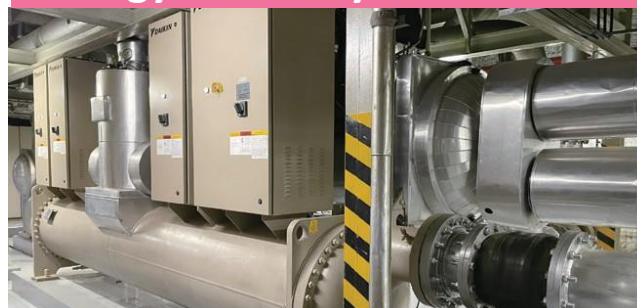
Chiller & Air Conditioner & Solar Power (Indonesia) Yuko Keiso Co., Ltd.
