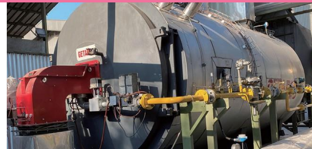
Thermal Oil Heater System (Indonesia) Fumakilla Limited
