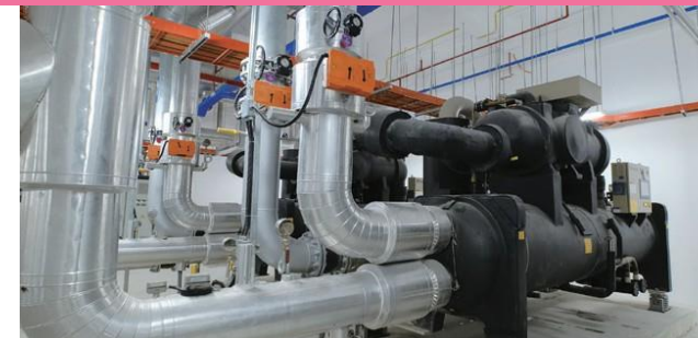
Chiller & LED Lighting (Vietnam) Tokyu Corporation
