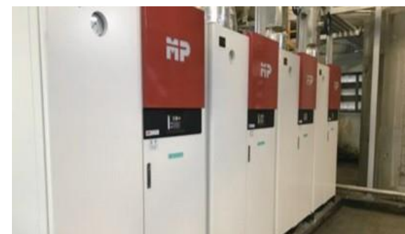
Introduction of High Efficiency Once Through Boiler to Garment Factory, Osaka Gas Co., Ltd., Thailand
