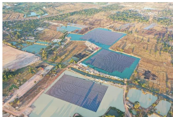
Floating Solar PV, TSB Co., Ltd., Thailand
