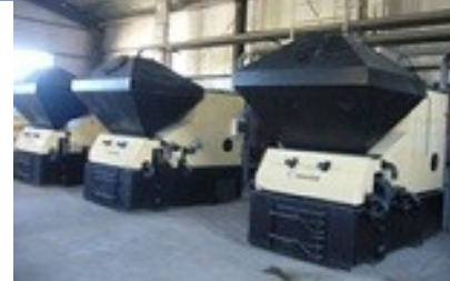
High-efficiency Heat only Boilers, Suuri-Keikaku, Mongolia
