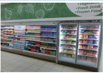
Energy saving at convenience stores, Panasonic, Indonesia
