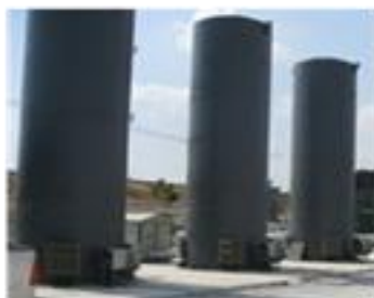
Excess LFG enters flares
