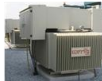
Generated electricity sent to local grid
