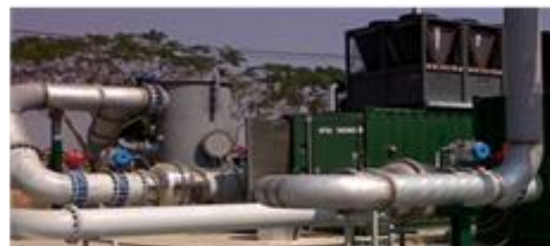
LFG enters pre-treatment plant
