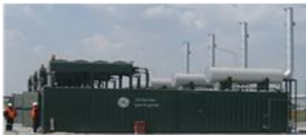
LFG sent to gas engines for electricity generation
