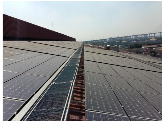
Factory building 798.72 kW
