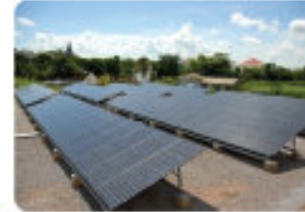
Micro-grid of PV and batteries
