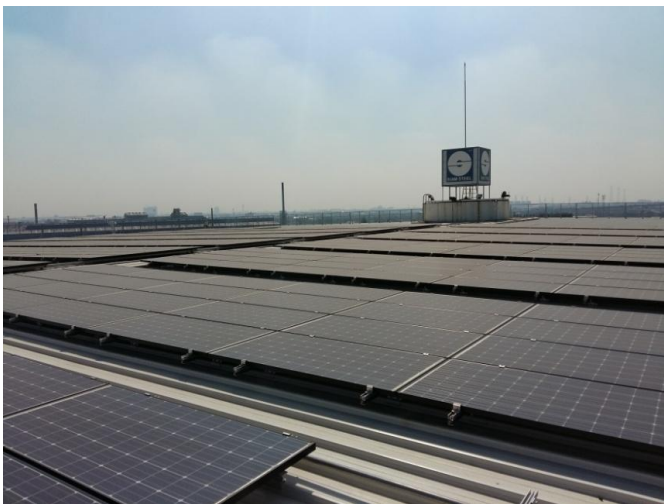
Office building 195.84 kW
